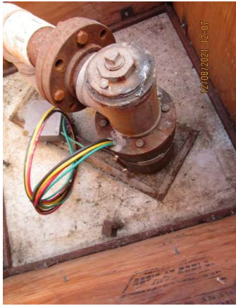
Well 1 With Sealed Wires
