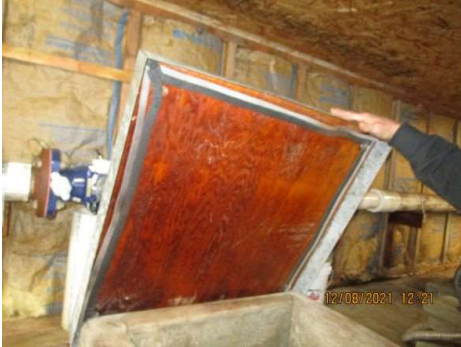
Large Storage Tank Hatch Gasket
