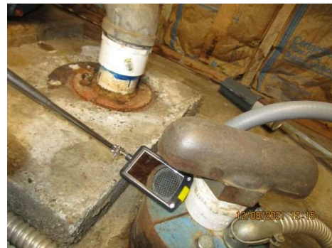
Small Storage Tank Vent
