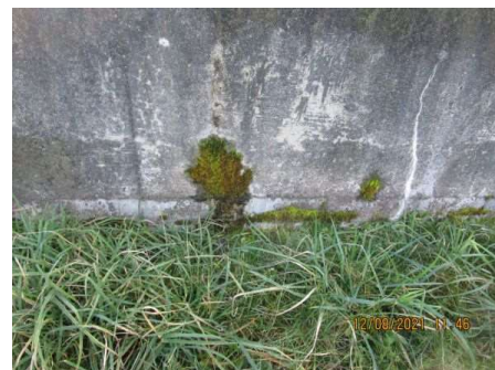
North Side Large Storage Tank
