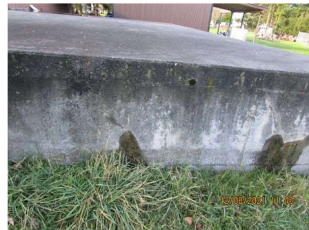
East Side Large Storage Tank
