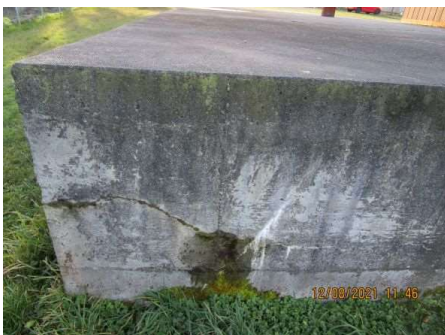
North Side Large Storage Tank
