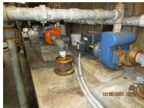
Booster Pumps for Small Storage Tank
