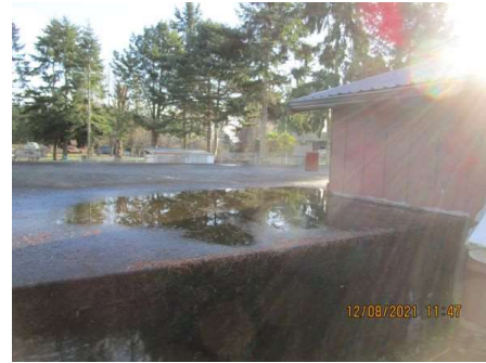
Large Storage Tank - Ponding
