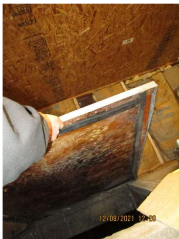
Small Storage Tank Hatch Gasket
