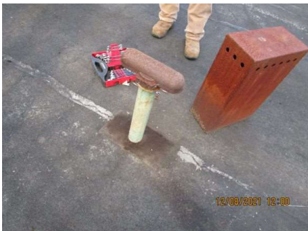
Large Storage Tank Vent
